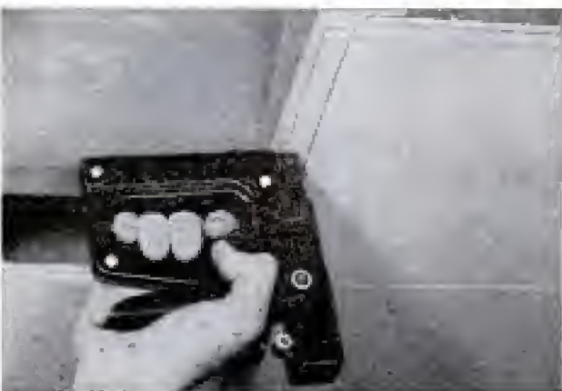
When it comes to fastening ceiling tile in place, a stapler does a neat job without marring surface
